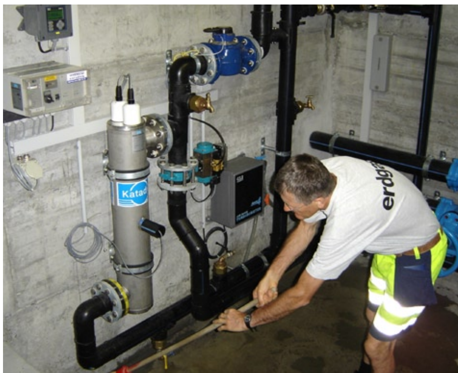
UV water treatment plant Burg Hard
